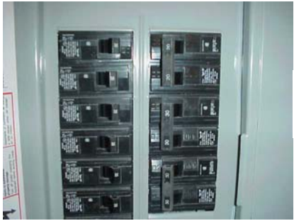
Circuit Breaker Box
