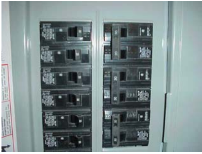
Circuit Breaker Box
