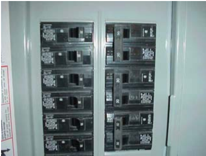
Circuit Breaker Box
