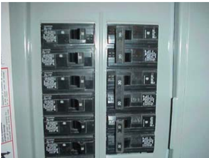
Circuit Breaker Box
