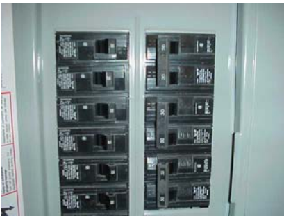
Circuit Breaker Box
