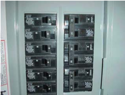
Circuit Breaker Box
